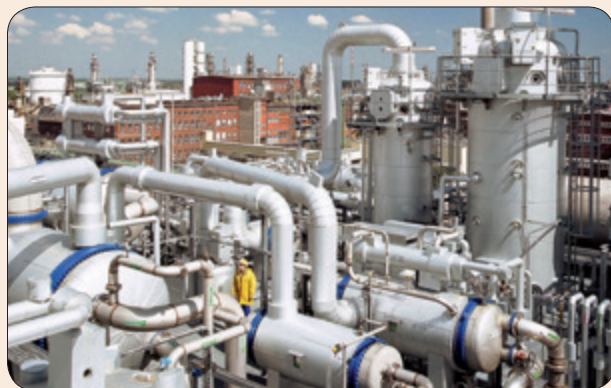
Fig. 4: Citral plant at BASF Ludwigshafen site as an example for applied reaction and process engineering. Citral is a key chemical intermediate to produce fine chemicals like vitamins, fragrances or aroma-chemicals (source: BASF SE).
